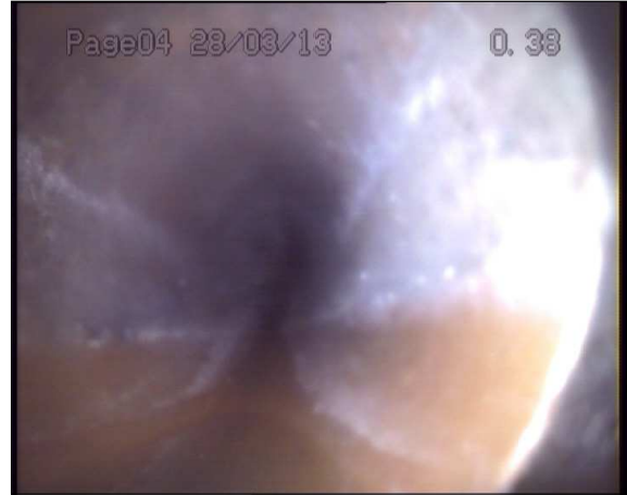
Photo: 3_3_31_A.jpg 0.3m, Shape of sewer changes at this point
