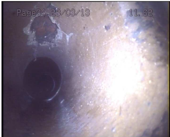
Photo: 1_1_18_A.jpg 11.7m, Hole in sewer, from 12 to 1 o'clock
