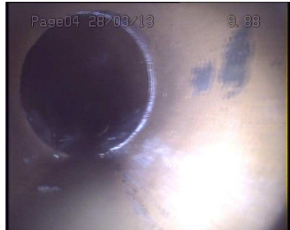
Photo: 1_1_13_A.jpg 10m, Joint displaced, medium (between 1.0 and 1.5 times the pipe wall thickness)
