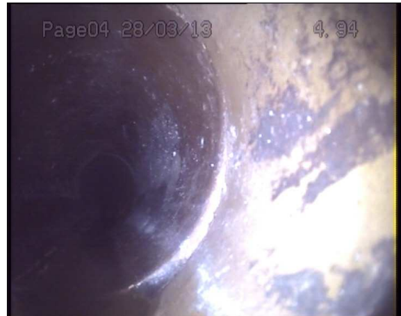
Photo: 1_1_9_A.jpg 5.1m, Joint displaced, medium (between 1.0 and 1.5 times the pipe wall thickness)
