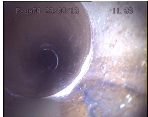
Photo: 1_1_19_A.jpg 12m, Joint displaced, medium (between 1.0 and 1.5 times the pipe wall thickness)
