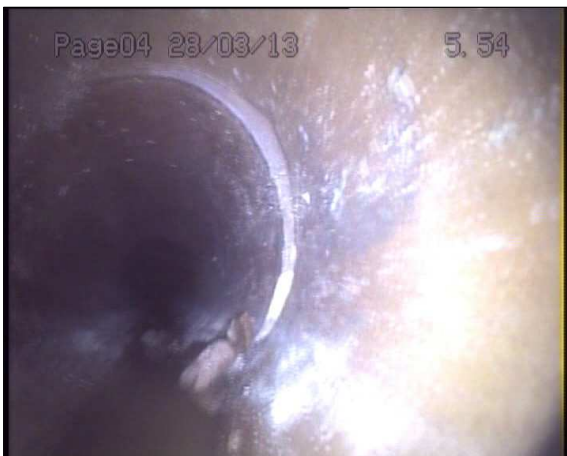
Photo: 1_1_10_A.jpg 5.7m, Joint displaced, medium (between 1.0 and 1.5 times the pipe wall thickness)
