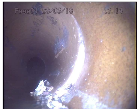
Photo: 1_1_21_A.jpg 13.2m, Joint displaced, medium (between 1.0 and 1.5 times the pipe wall thickness)
