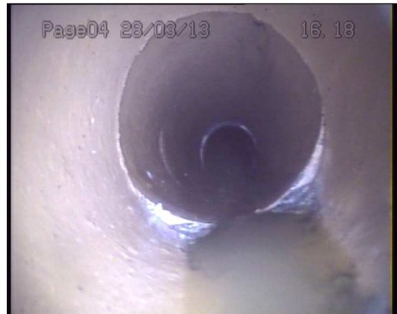
Photo: 1_1_25_A.jpg 16.1m, Joint displaced, medium (between 1.0 and 1.5 times the pipe wall thickness)
