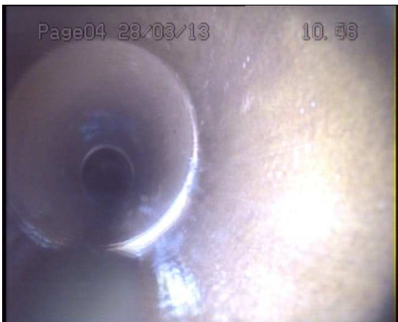
Photo: 1_1_15_A.jpg 10.4m, Joint displaced, medium (between 1.0 and 1.5 times the pipe wall thickness)
