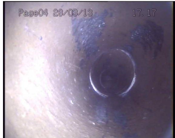
Photo: 1_1_27_A.jpg 17.1m, Joint displaced, medium (between 1.0 and 1.5 times the pipe wall thickness)
