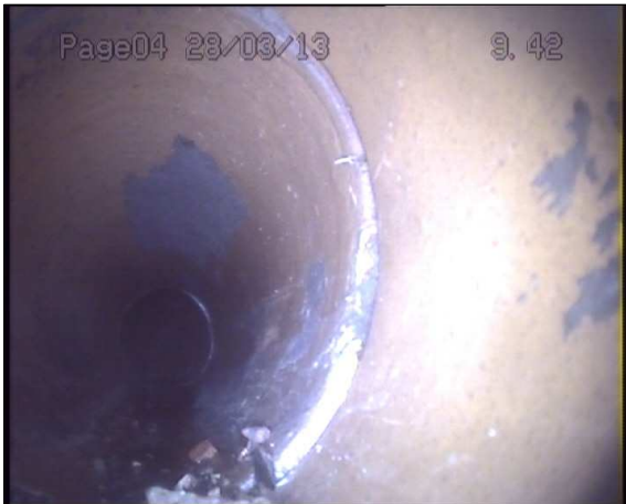
Photo: 1_1_12_A.jpg 9.5m, Joint displaced, medium (between 1.0 and 1.5 times the pipe wall thickness)
