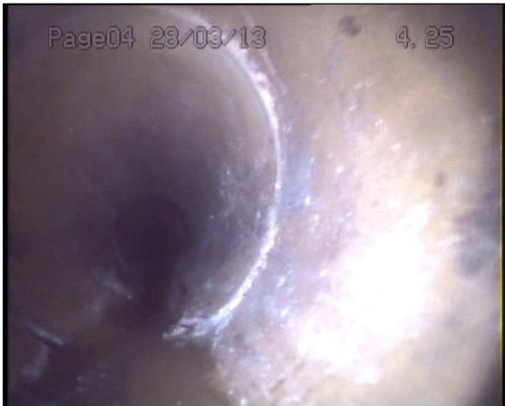
Photo: 1_1_8_A.jpg 4.4m, Joint displaced, medium (between 1.0 and 1.5 times the pipe wall thickness)
