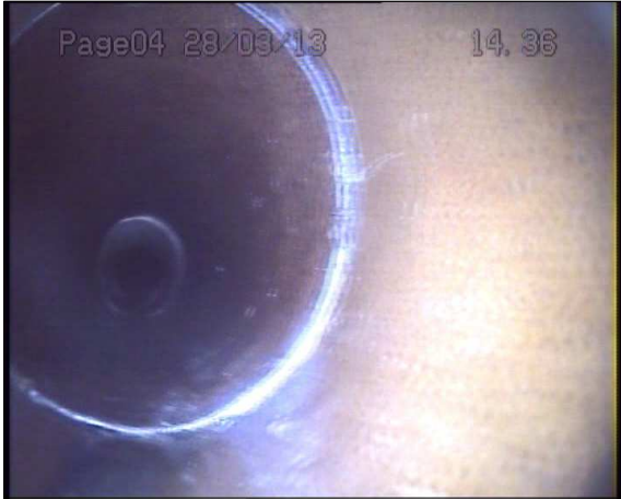
Photo: 1_1_22_A.jpg 14.3m, Joint displaced, medium (between 1.0 and 1.5 times the pipe wall thickness)
