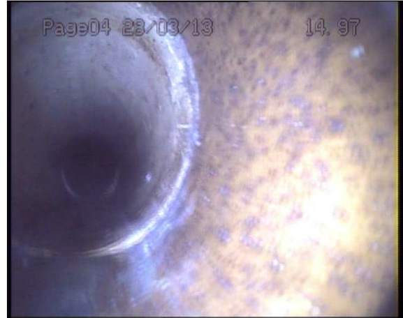
Photo: 1_1_23_A.jpg 15m, Joint displaced, medium (between 1.0 and 1.5 times the pipe wall thickness)
