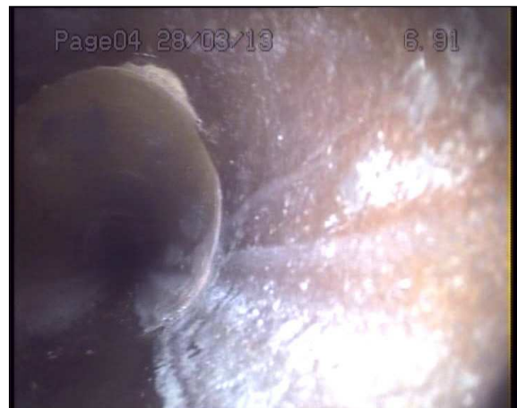
Photo: 1_1_11_A.jpg 6.9m, Joint displaced, medium (between 1.0 and 1.5 times the pipe wall thickness)
