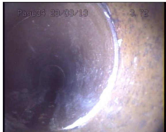
Photo: 1_1_7_A.jpg 3.8m, Joint displaced, medium (between 1.0 and 1.5 times the pipe wall thickness)
