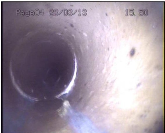
Photo: 1_1_24_A.jpg 15.6m, Joint displaced, medium (between 1.0 and 1.5 times the pipe wall thickness)
