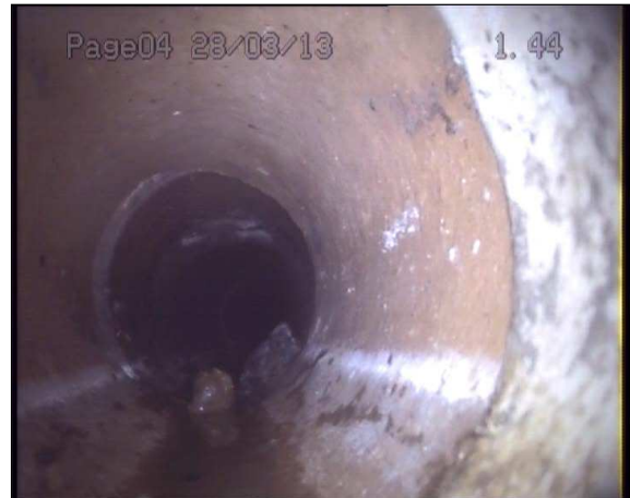
Photo: 1_1_4_A.jpg 1.9m, Sewer material changes
