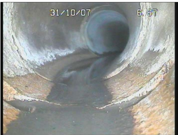
Photo: 85b, Tape No.: DVD, 00:00:00 6.6m, Circumferential Crack, from 03 to 09 o'clock
