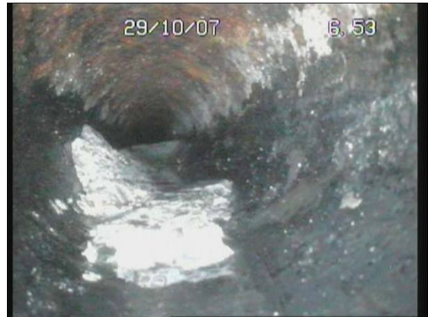
Photo: 20a, Tape No.: DVD, 00:00:00 6.5m, Obstruction (Concrete/Tarmac), 40% cross-sectional area loss
