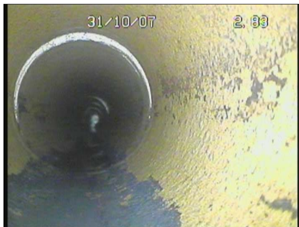
Photo: 77a, Tape No.: DVD, 00:00:00 2.8m, Joint displaced. Medium
