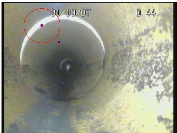
Photo: 24_2a, Tape No.: DVD, 00:00:00 0.4m, Joint displaced. Medium
