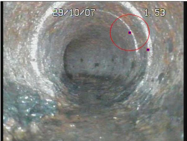
Photo: 5_2a, Tape No.: DVD, 00:00:00 1.5m, Circumferential Crack, from 12 to 03 o'clock
