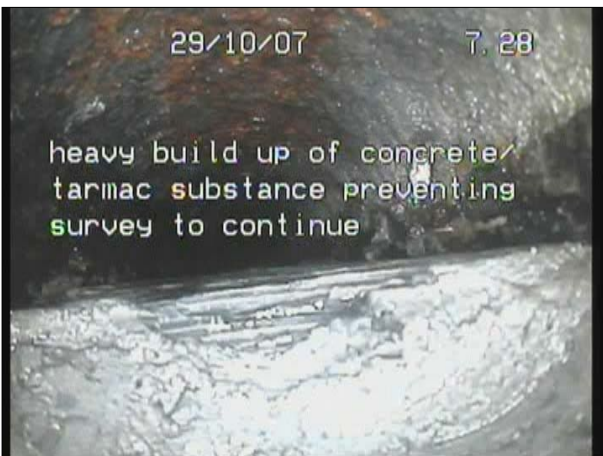
Photo: 21a, Tape No.: DVD, 00:00:00 7.2m, Obstruction (Concrete/Tarmac), 50-60% cross sectional area loss
