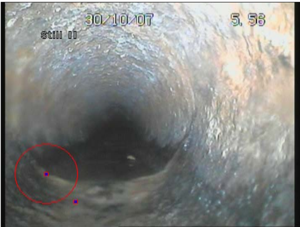
Photo: 14_2a, Tape No.: DVD, 00:00:00 5.5m, Joint displaced. Medium
