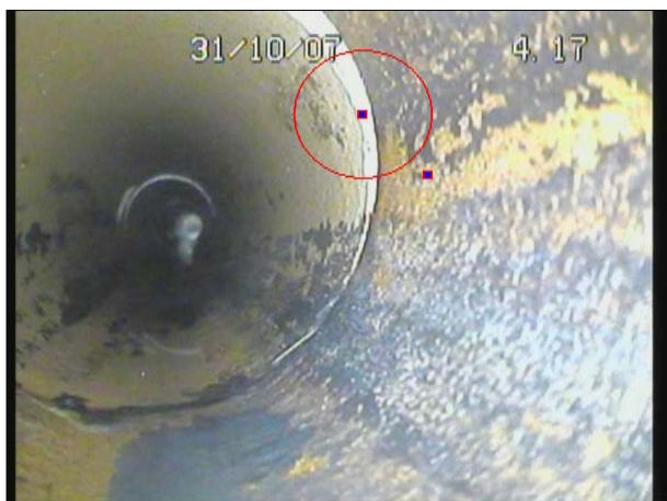
Photo: 24_5a, Tape No.: DVD, 00:00:00 4.8m, Joint displaced. Medium
