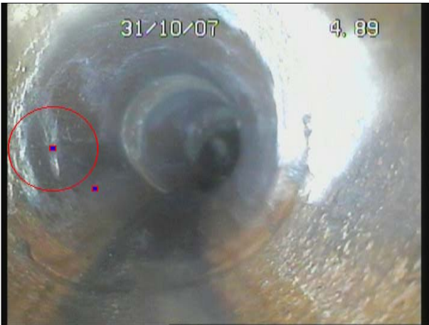
Photo: 25_2a, Tape No.: DVD, 00:00:00 4.8m, Longitudinal Crack, at 09 o'clock
