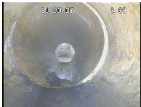
Photo: 79a, Tape No.: DVD, 00:00:00 6.6m, Joint displaced. Medium
