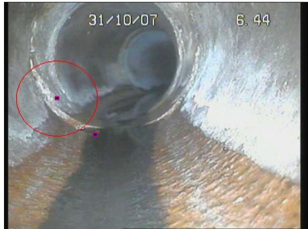
Photo: 25_4a, Tape No.: DVD, 00:00:00 6.6m, Circumferential Crack, from 03 to 09 o'clock
