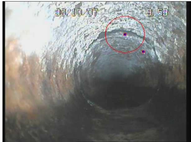
Photo: 14_3a, Tape No.: DVD, 00:00:00 9.5m, Joint displaced. Medium
