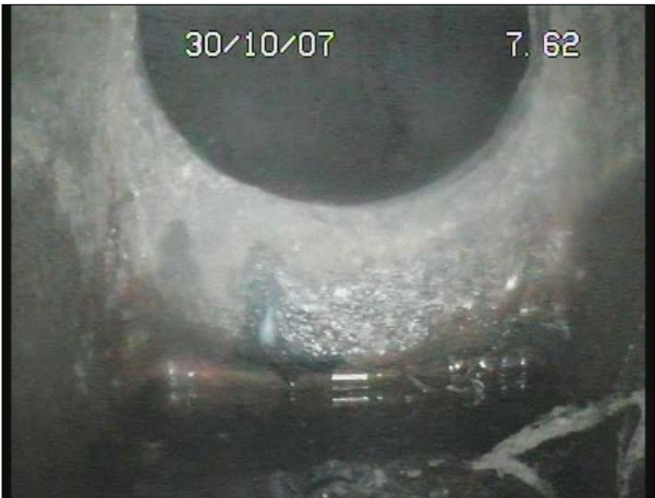
Photo: 36a, Tape No.: DVD, 00:00:00 7.6m, Finish Survey, Remark: Possibly 100mm Stack pushed into 150mm Main Line
