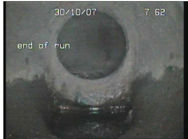
Photo: 36b, Tape No.: DVD, 00:00:00 7.6m, Finish Survey, Remark: Possibly 100mm Stack pushed into 150mm Main Line
